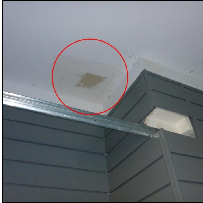
Patched in garage
