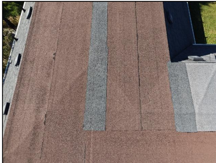
Patched flat roof
