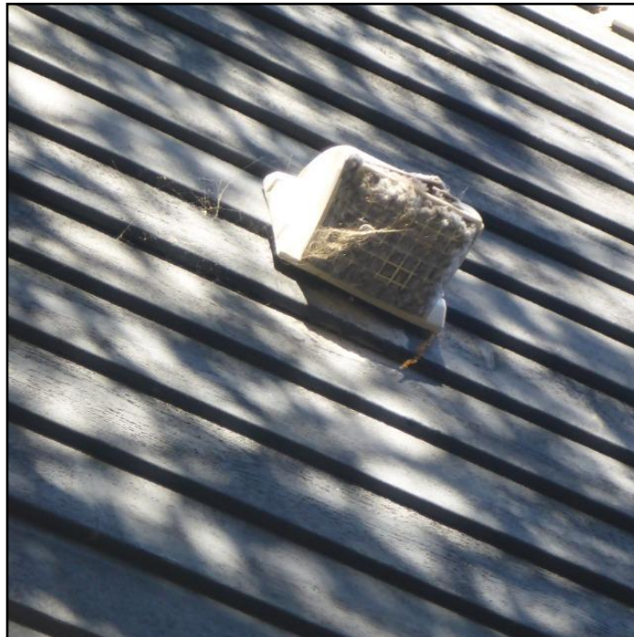
Plugged dryer vent
