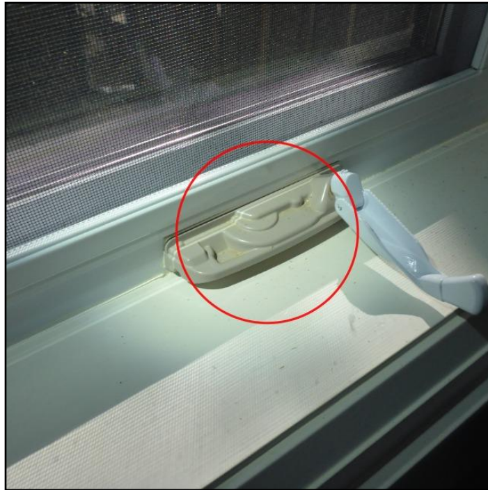
Missing cover in dining room
