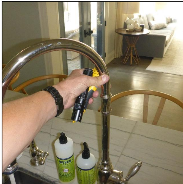
Loose at kitchen
