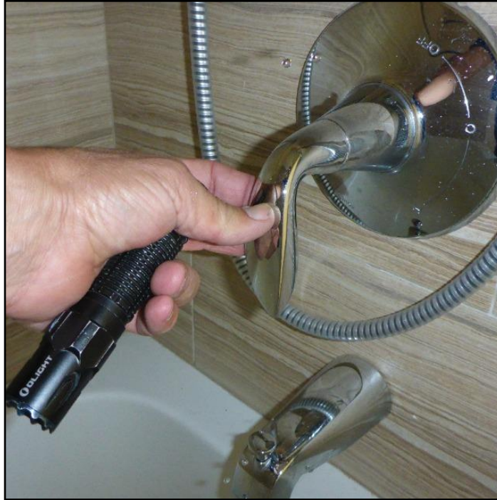
Loose handle at tub
