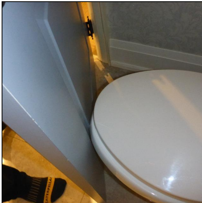
Missing door stop in powder room
