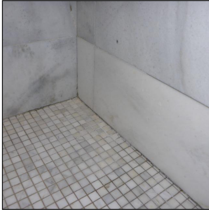
Shower stall maintenance required
