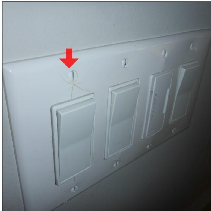
Cracked at primary ensuite
