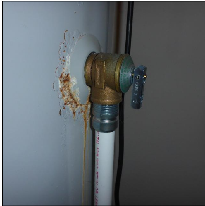
Corroded water heater
