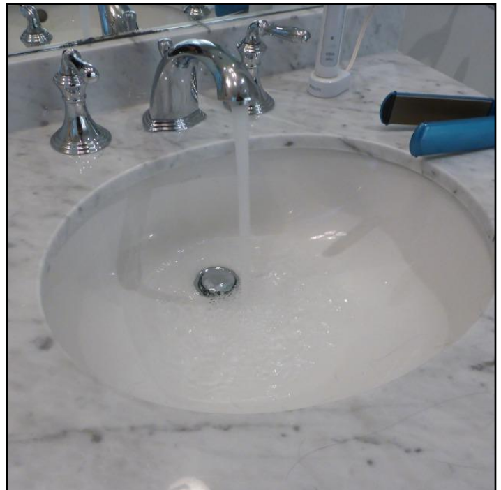
Slow drain at primary ensuite
