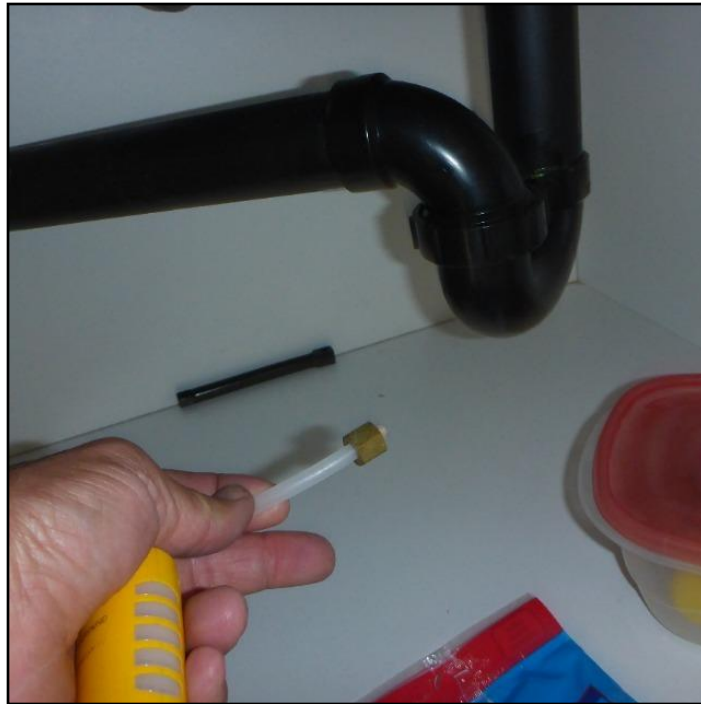
Disconnected at laundry room
