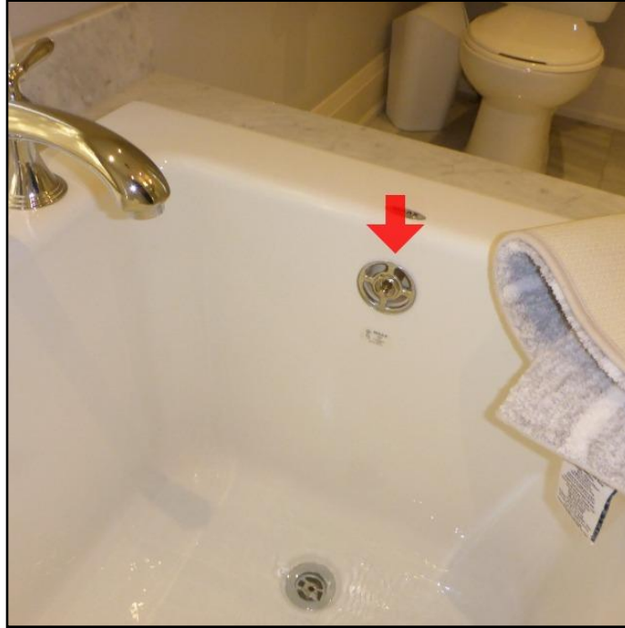
Missing cover in primary ensuite
