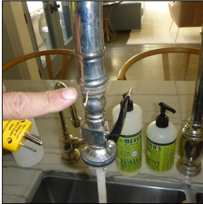
Leak at kitchen
